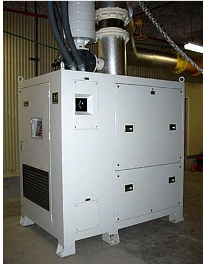
Neuros Blower at the Lakota Wastewater Treatment Plant
