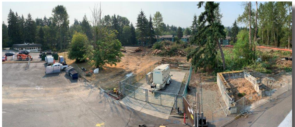
The site location has been cleared in preparation for the new headquarters building and parking lot.
